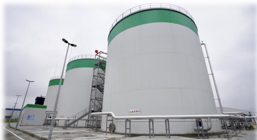
Kemberburgaz Biomethanization Facility
