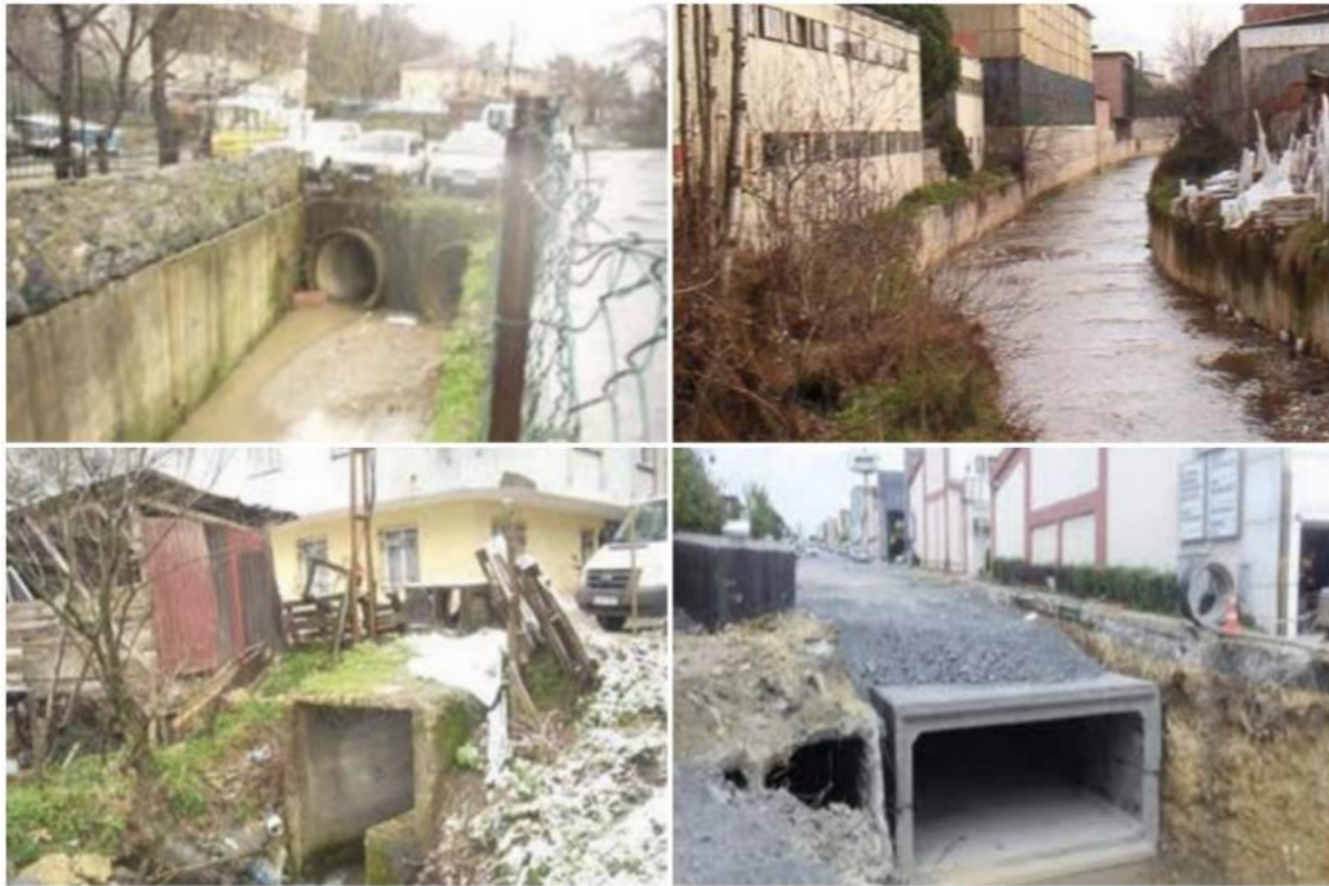
Figure 30. Examples of narrowed and reclaimed stream channels. In fact, the stream channel was not rehabilitated, on the contrary, it was concreted. Rehabilitation works carried out in this way trigger flood disasters during heavy rain events.
